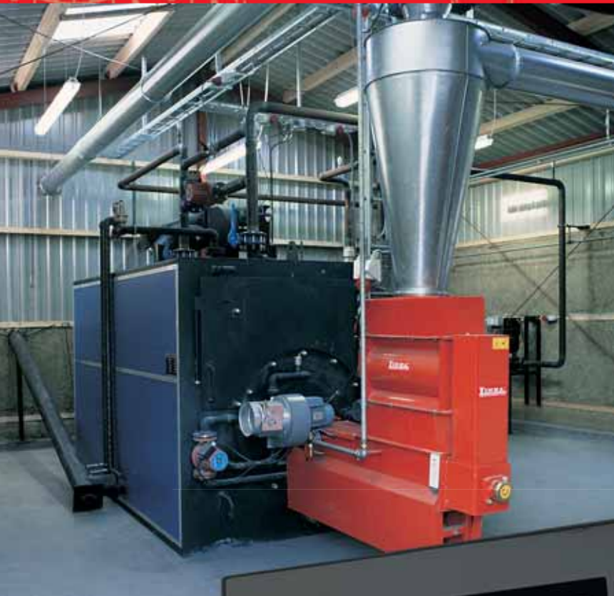
Cyclone and boiler system
